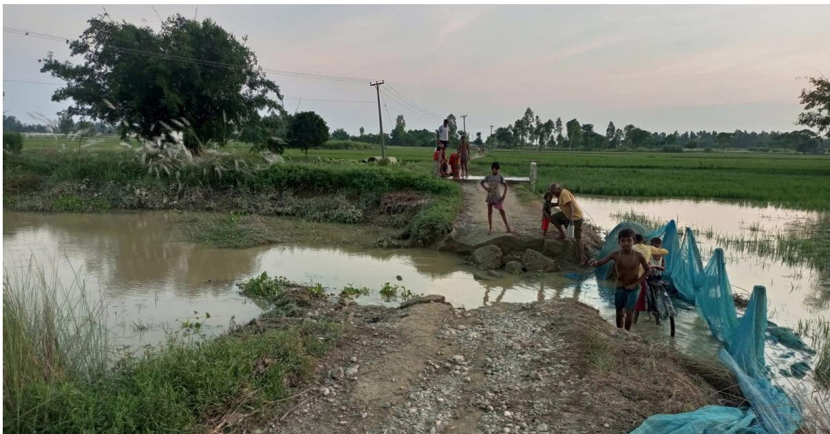
Road connecting Jingadwa Belchhuwa village to other areas got damaged due to flooding
